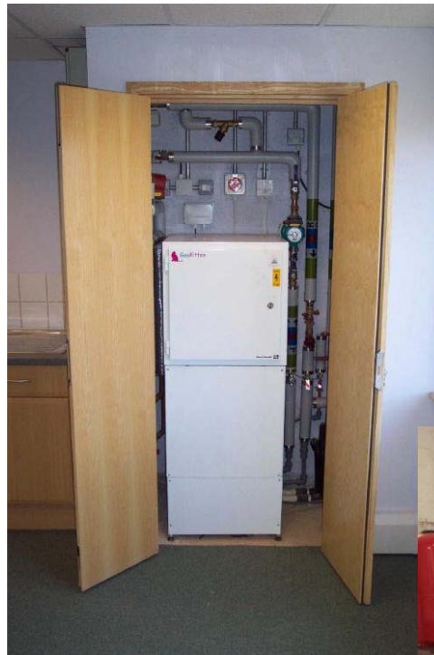
Kensa heat pump Blackhall Mill community centre
